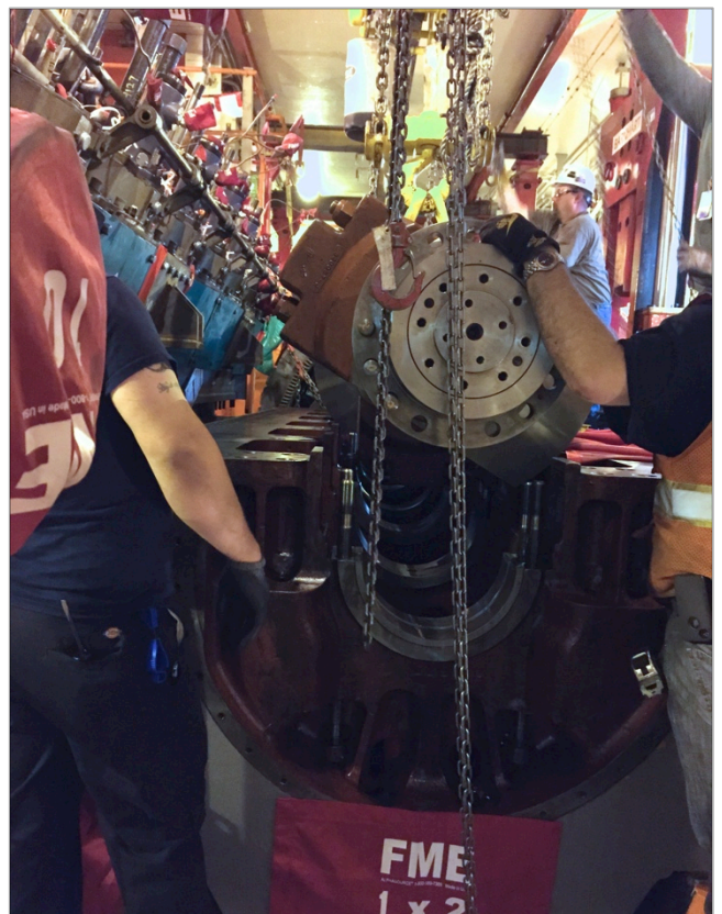
Rigging of damaged crankshaft from the engine
