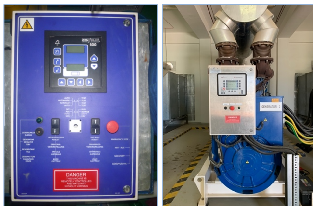
Legacy Panel (left) and Upgrade Panel (right)
