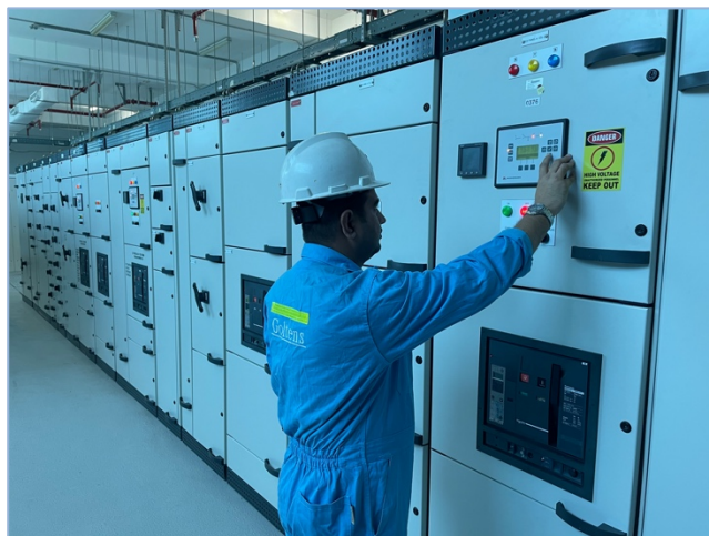
ATS Panels after upgrade of system
