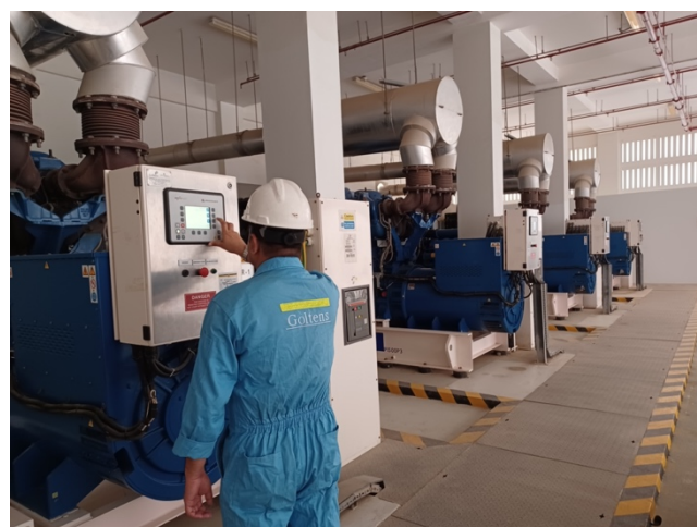
Configuration of controls on engine after installation
