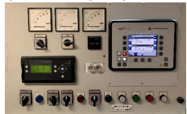
Figure 3: Panel after upgrade
