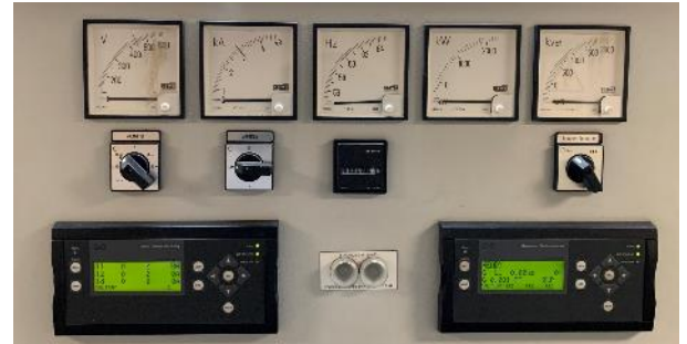
Figure 1: Panel before upgrade
