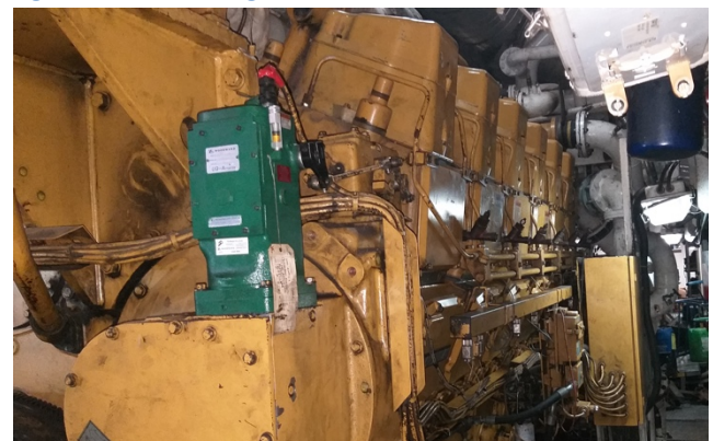
Figure 4: Main Engine with UG Actuator
