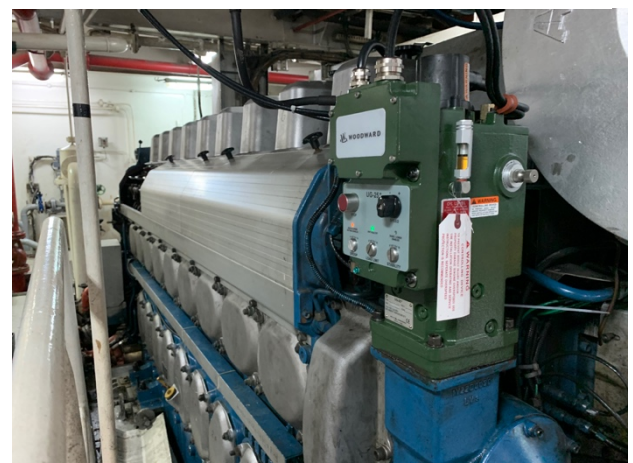
Figure 3: Woodward UG25+P3 after retrofit
