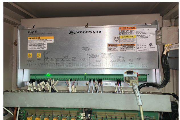
Figure 3: Digital Woodward 2301E LSSC installed
