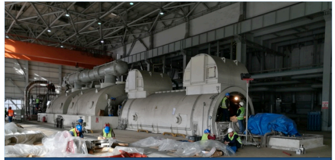
Number one Steam Turbine Generator
