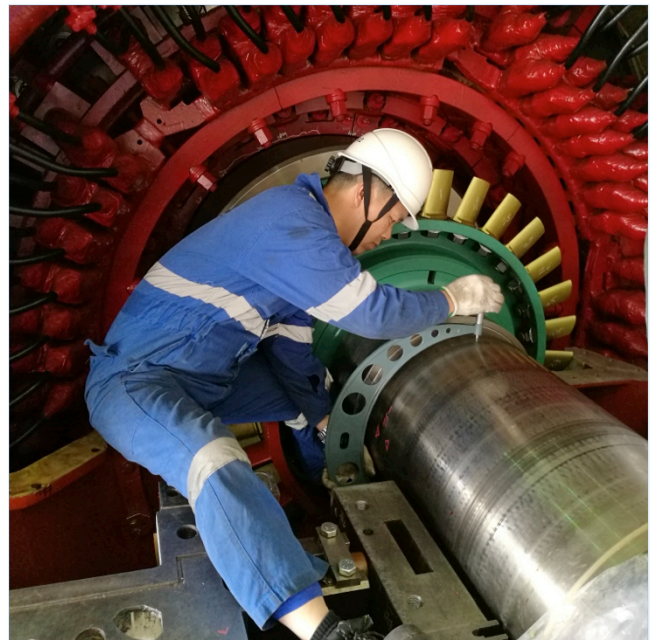
Complete inspection of turbine journal
