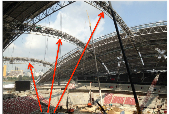
Location of winches high above stadium floor
