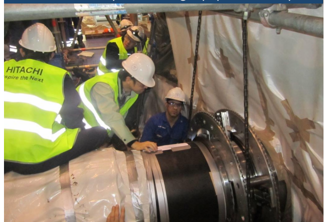
Manufacturer reps observing equipment set up
