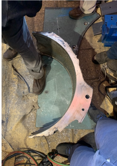
Figure 5: half of shaft seal liner removed
