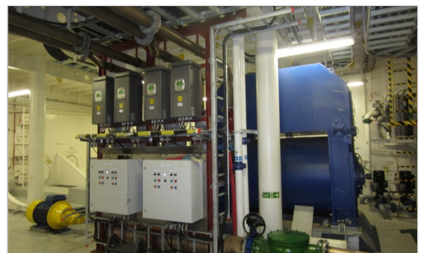
Main Engine cooling system installed
