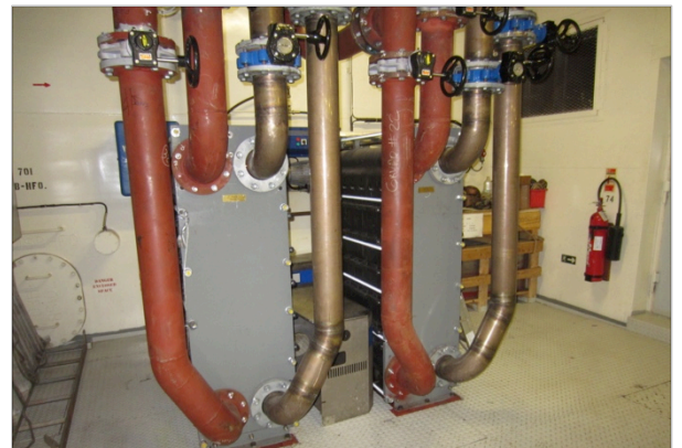
Main Engine cooling system installed
